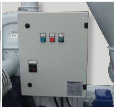
Control cabinet for automatic starting/stopping the motor.
